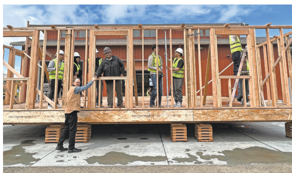
Architect Thomas Rettenwender (below) and Rancho Cielo construction students with the Nexus 01 home in progress.
